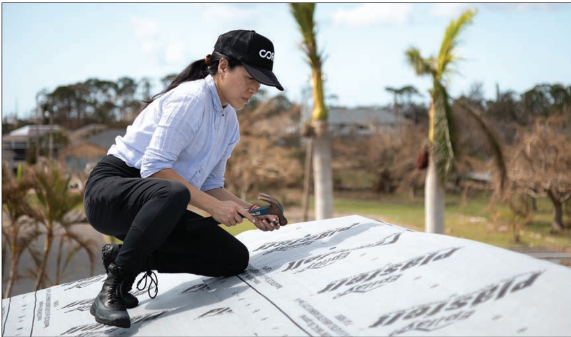
Ann Lee tarps a roof near Fort Myers, Florida during the initial phase of CORE's response to Hurricane Ian in 2022
