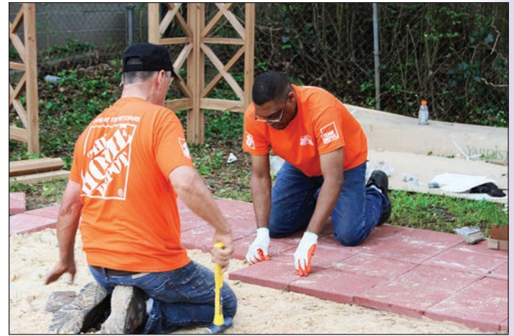
Team Depot volunteers created an outdoor patio for an Atlanta-based Vietnam Army veteran, one of 500 veterans to receive home repairs from The Home Depot on a single day in September 2014.
