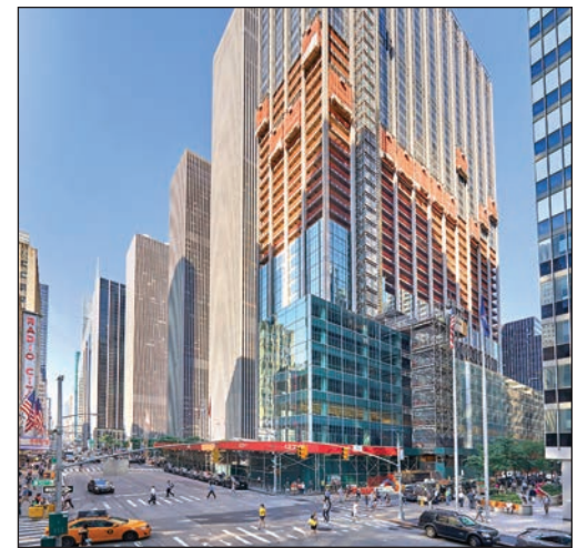
1271 Avenue of the Americas, which Rockefeller Group is in the process of redeveloping as part of a $600 million project.
