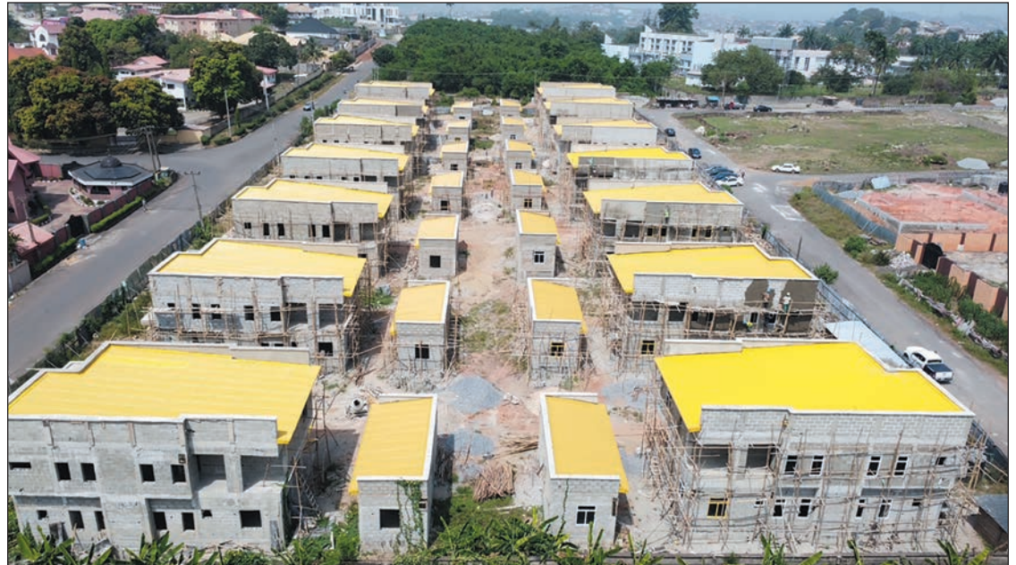
Aerial view of the ongoing detached duplex project at the Ibara Housing Estate, Abeokuta Ogun State, Nigeria by Still Earth Construction
