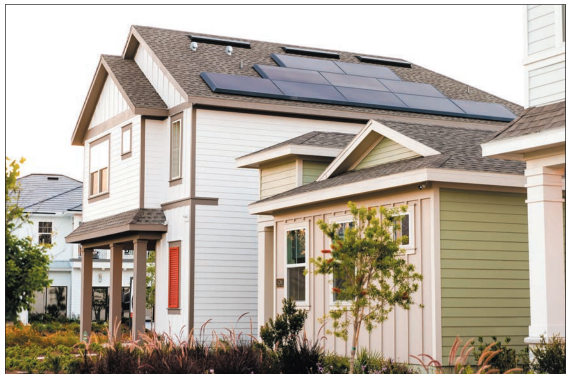
Solar panel installation at Sunbridge, Tavistock's second master-planned community in Central Florida
